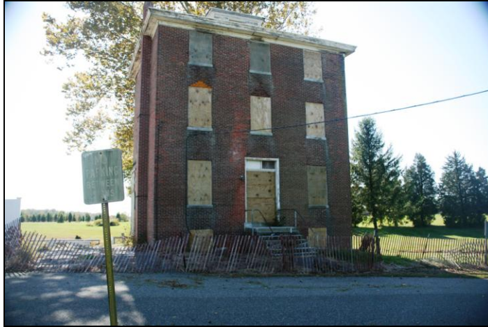
Figure 2.2. Salem County Asylum, October 19, 2009 3:55 PM. The almshouse was demolished due to water damage. Courtesy of Irene Wanner, Salem County Public Information Assistant
